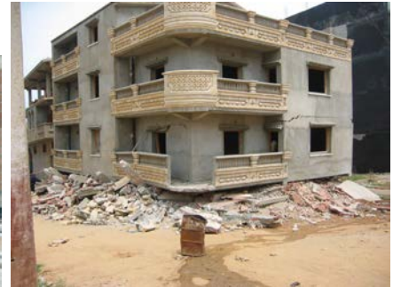
Figure 10: Typical earthquake damage: building collapse due to the soft storey effect (2003 Boumerdes earthquake)
