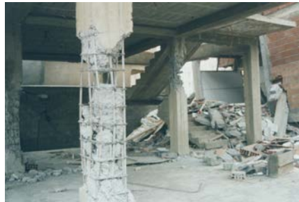
Figure 9: Seismic deficiencies - very poor quality of concrete (2003 Boumerdes earthquake)
