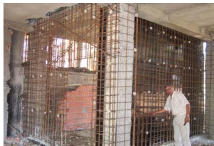
Figure 13: Seismic strengthening techniques: jacketing of columns and construction of new shear walls in the two directions (after the 2003 Boumerdes earthquake)
