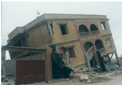
Figure 11: Typical earthquake damage: soft storey collapse (2003 Boumerdes earthquake)
