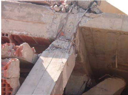
Figure 8: Seismic deficiencies: weak beam-column joint (2003 Boumerdes earthquake)
